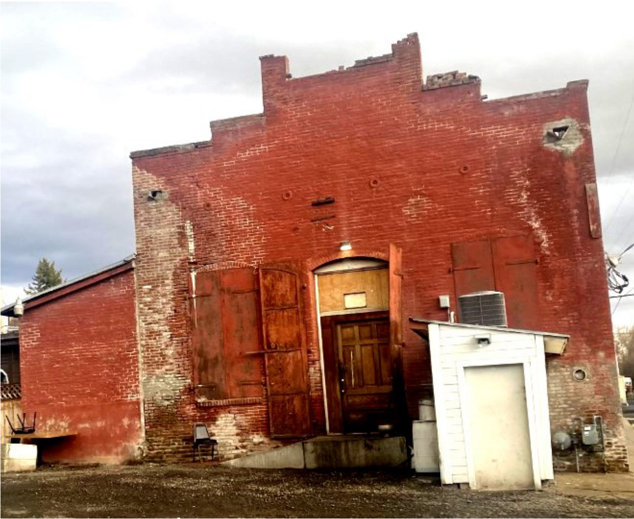
Right: North Wall of building. Note steel shutters at the back door and windows on either side of the back door. Contractor will be repairing the large shutters.
