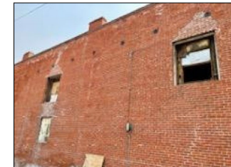
West Wall needs brick work.
